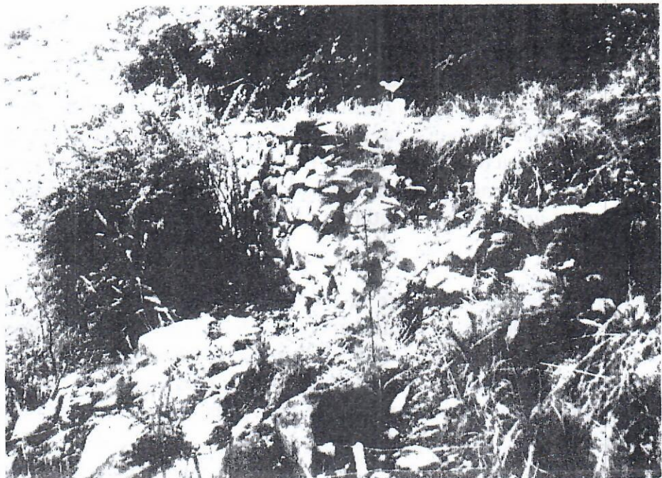
I.14 Stone Wall: This extensive stone retaining wall, at the intersection of the Terrace and Dogwood Walk & Meadows requires reconstruction. LANDSCAPES
